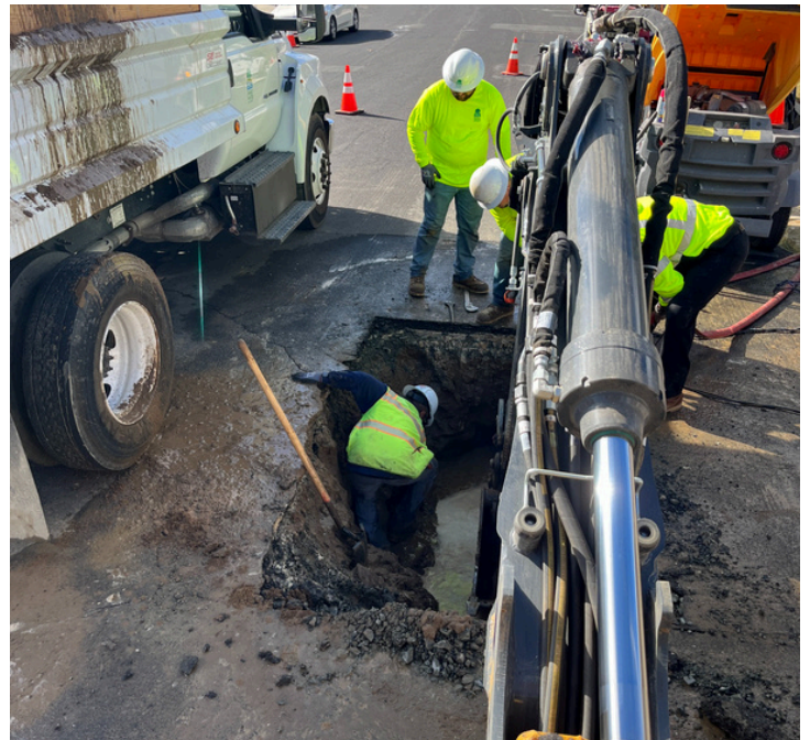
Diablo Water District performs all water main and service line repairs in-house.
